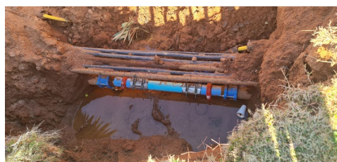
Failed AC Pipe replacement
