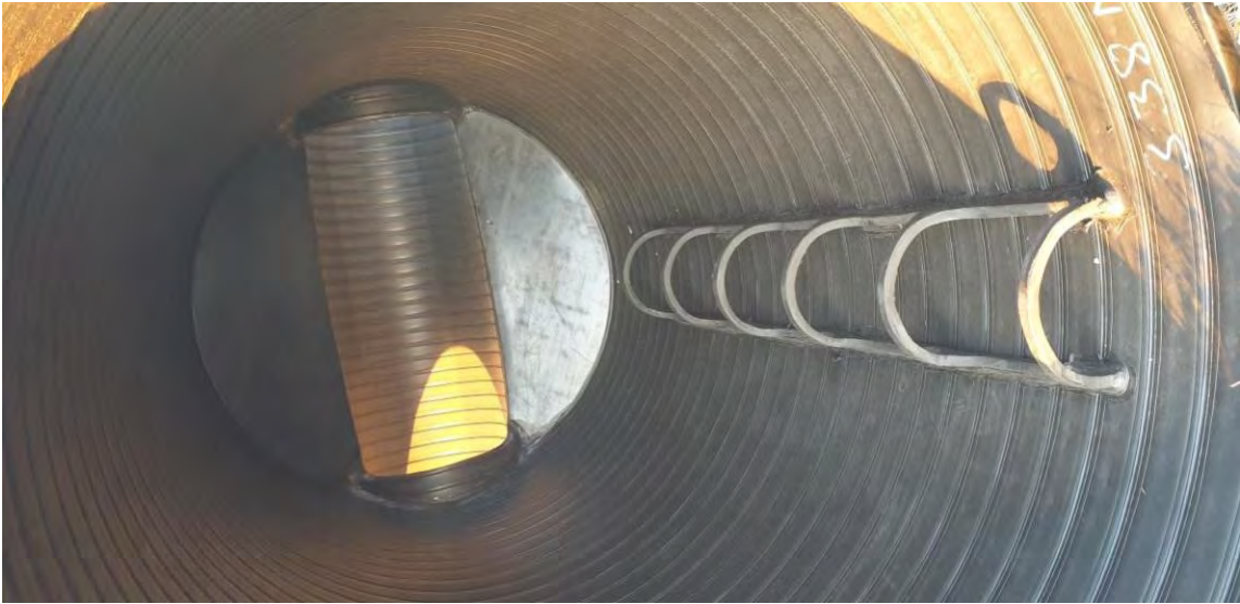
Inside view of Benching & Ladder
